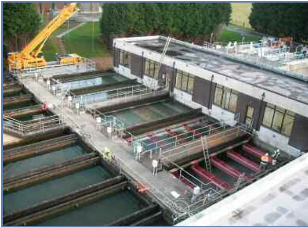
Clareville Water Treatment Plant, Limerick
