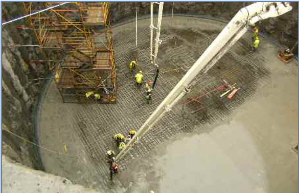
Mullingar Wastewater Treatment Plant
